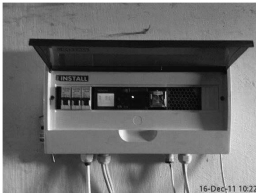
Picture 2. Control unit
