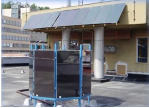
Figure 2.1.1 The Photovoltaic test site
